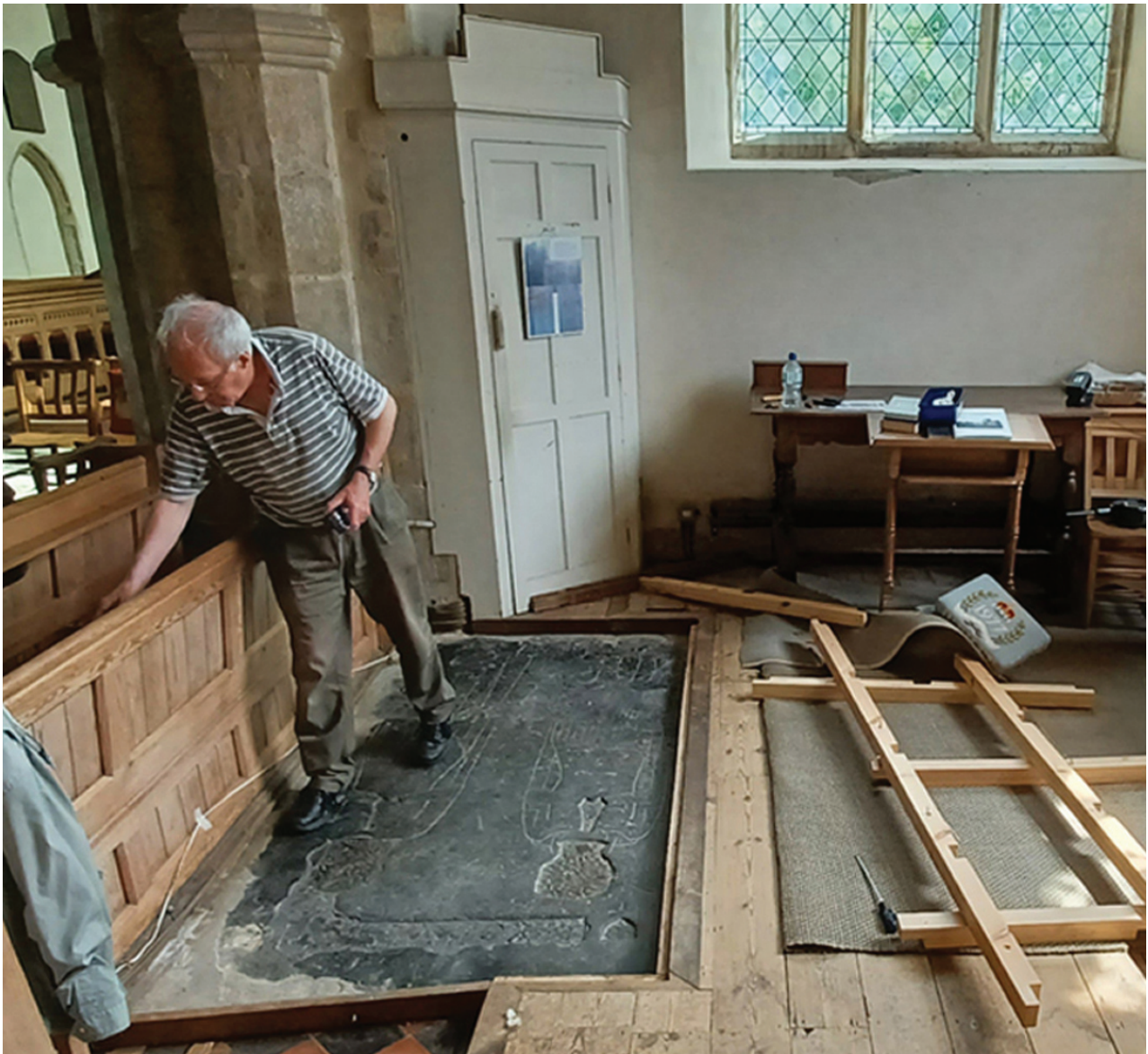
Fig.3. Dismantling the woodwork at Gressenhall to enable full recording of the Flemish slab, May 2022. (photo: © Frank Wheaton)
