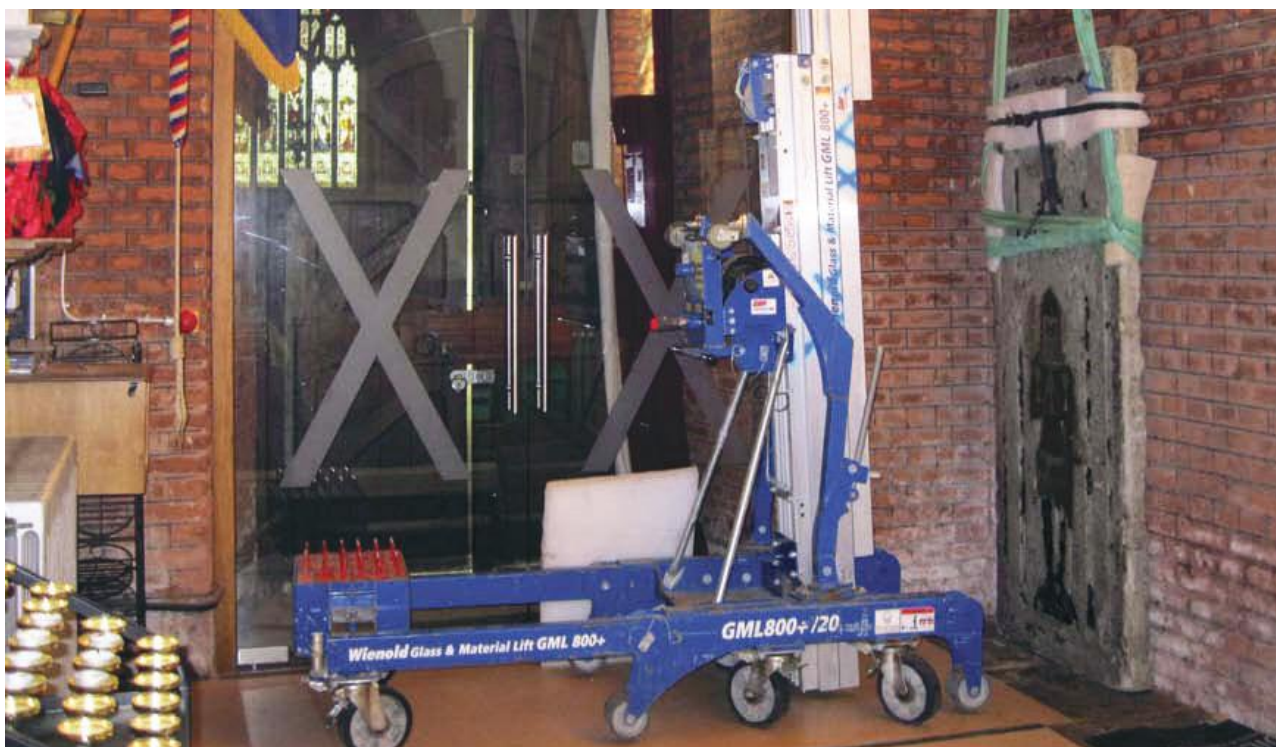
The Stapel brass and slab being hoisted into position in Rochford church.
