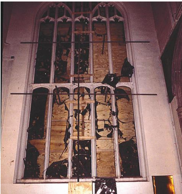
Damage to the west window in 1992 (photo: Stephen Freeth)
