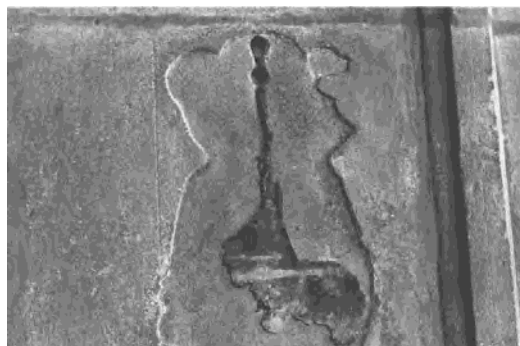
FIG. 31 Detail of Stafford monument at Blatherwyck: showing how lead was poured through holes in the slab from behind
